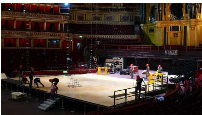
Harlequin Liberty® floor installation at the Royal Albert Hall. Panels had to be cut on-site to accommodate the iconic elliptic curve of the stage.
